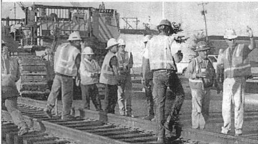
On day 2 of the move, the Madame Queen was escorted down the center of South Grand St. on panel track. In this photo, Messer crew members have completed the linking of two panel track sections, and crew chief Daniel King signals to equipment operators.
