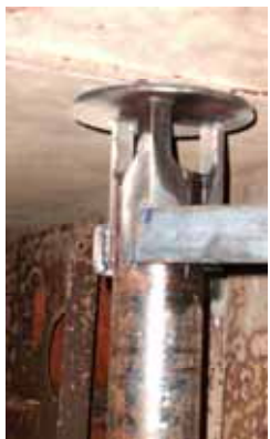
Diffuser top of standpipe
