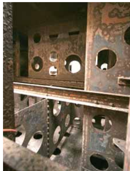
A view inside the tender showing the many baffles that inside workers had to deal with. The tender is entered through the hatch on top. Some welding was done more than 20 feet inside, behind several baffles.
