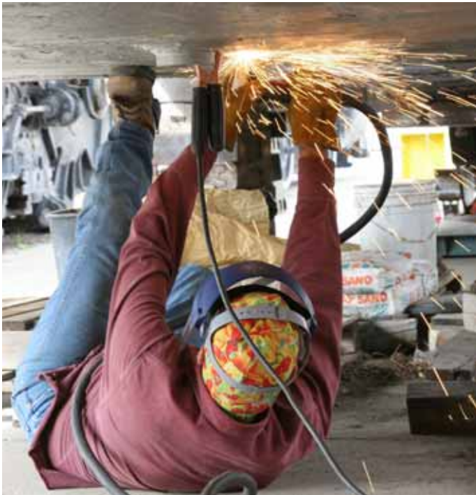
On his back with feet braced on the bottom of the tender, Lester Sanders of ABC Welding uses a plasma torch to cut a hole through the thick cast iron bottom of the tender.
