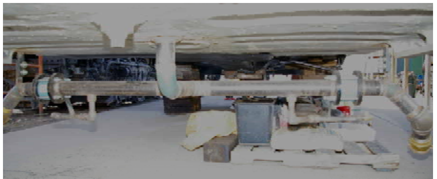
Trackside water system during installation, showing both side pipes and bottom of vertical standpipe. Picture was taken from rear of tender bottom looking forward.
