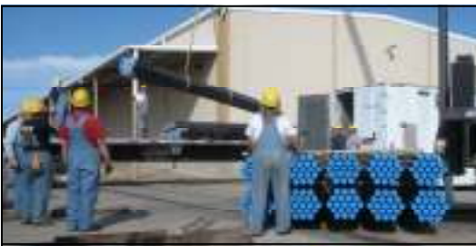
Crew members watch as a bundle of flue tubes is lifted from the truck to be placed atop the stack.
