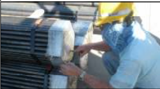
Randy McEntire counts individual super heater pipes. He inventoried and marked each bundle.
