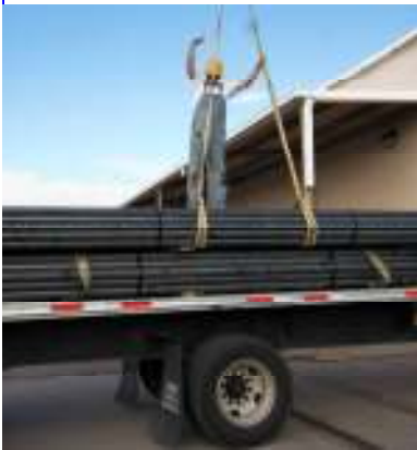
Unloading the new flue tubes and superheater pipes. Once the truck is in place, Rick Kirby signals to the crane operator to lift first bundle
