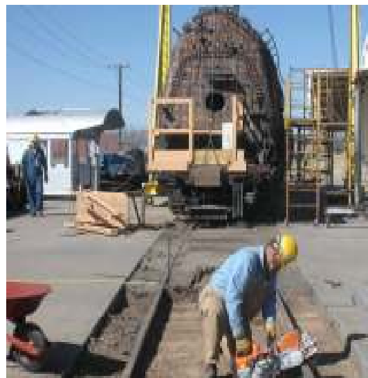
Preparing for pit construction. We needed a pit to access the undercarriage of 2926. Here, Jim Hills begins cutting the rails so the pit digging can begin. The finished and primed cab next to the locomotive is an example of Jim's fine restoration work.
